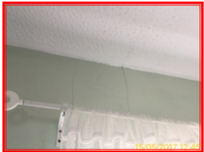
6.1.7 Pronounced settlement cracks to wall over window, advised by Alexandra majority are historic due to issue with loft storage. Photo's taken to measure change, if any going forward.
