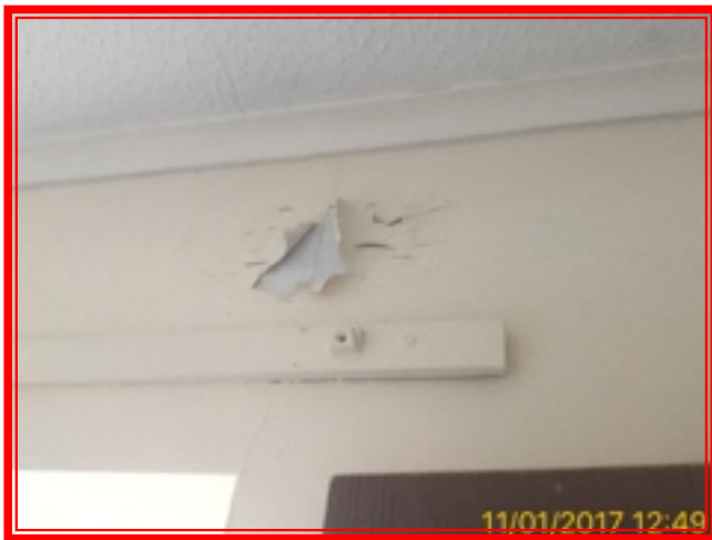
8.1.7 Paintwork has peeled above window, Alexandra has advised me since the extractor fan was fitted one year ago, this has not gotten any worse. Up to date photo added, remains in same condition.
