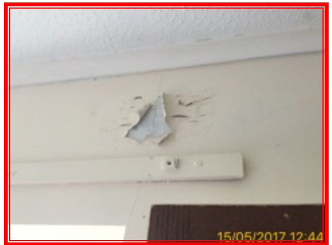
8.1.7 Paintwork has peeled above window, Alexandra has advised me since the extractor fan was fitted one year ago, this has not gotten any worse. Up to date photo added, remains in same condition.
