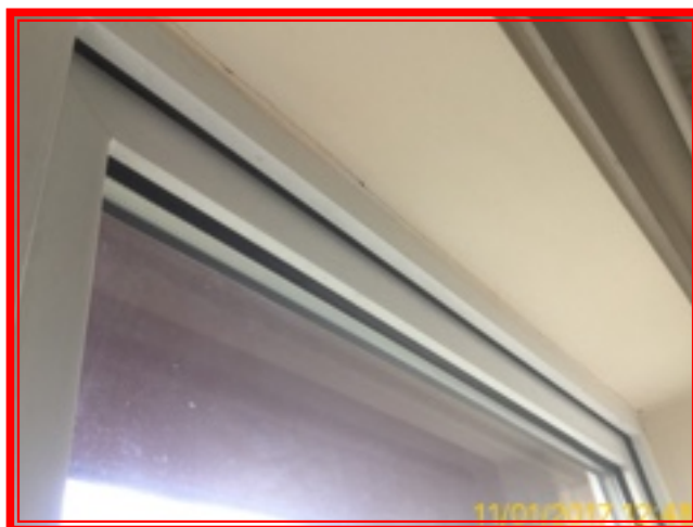
7.1.8 The window does not close flush, causing draft to edge. Noisy when opened. Issue remains.
